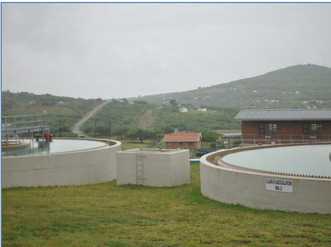
Figure 16.15 Photo of Middledrift WTP Clarifiers.
