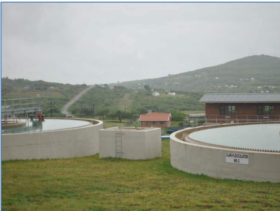
Figure 16.15 Photo of Middledrift WTP Clarifiers.
