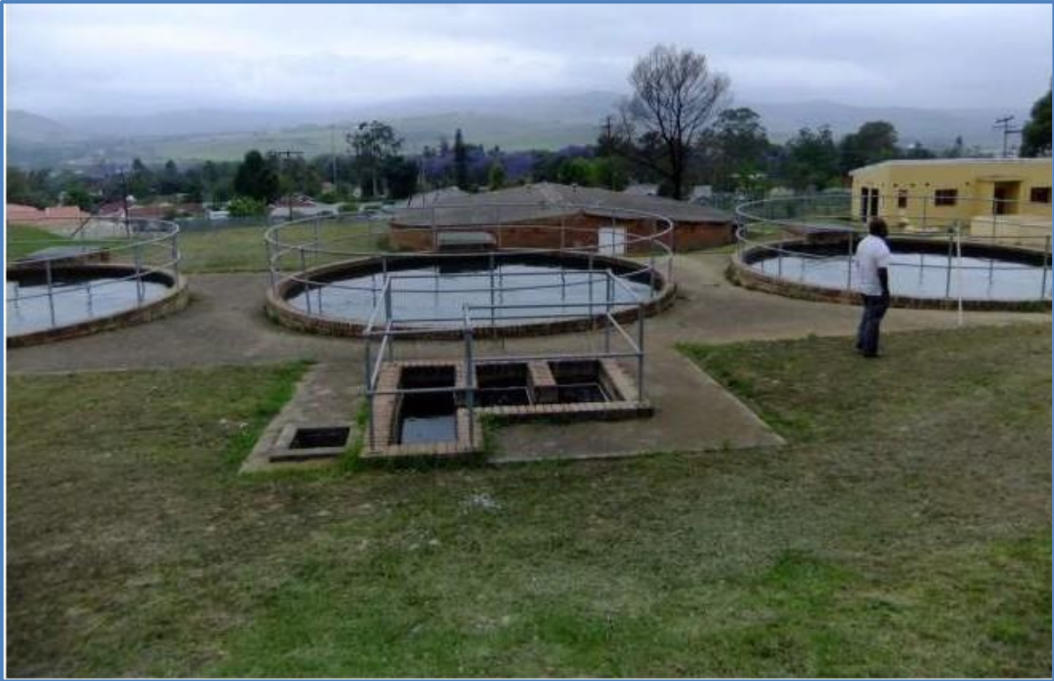
Figure 9.5 Pictorial view of the Mzimkhulu WTP
