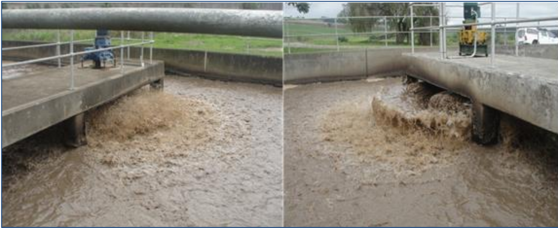
Figure 19.30 Different Mechanical Surface Aerators in Cool Air Reactor 1 and 2.
