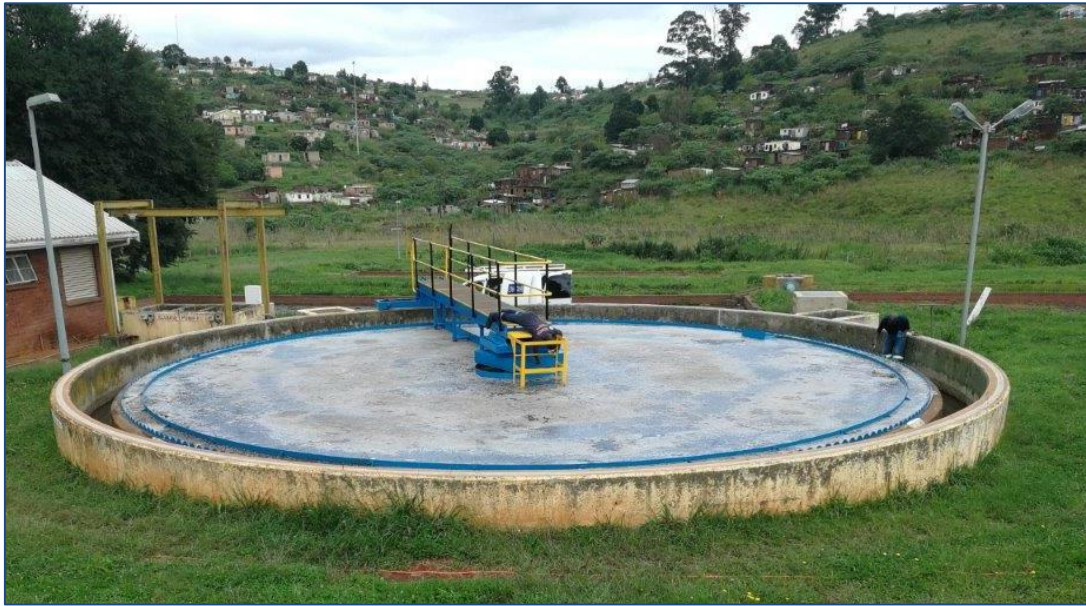
Figure 19.9 Clarifier No. 1 Ixopo WWW.
