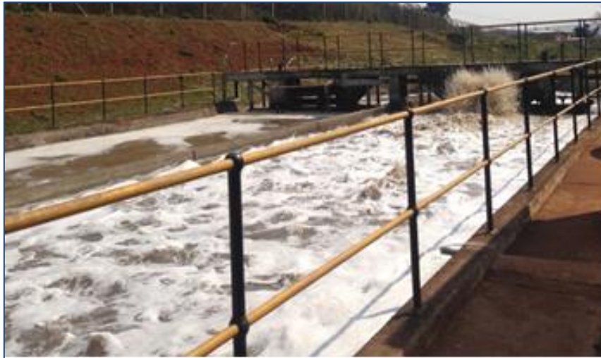
Figure 19.27 Appelsbosch WWT Oxidation Ditch (Aeration Tank).
