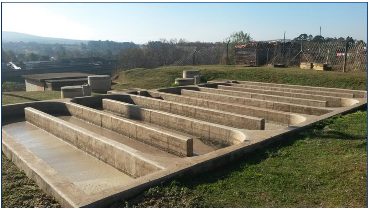
Figure 19.14 Howick WWW Chlorine Contact Tank.
