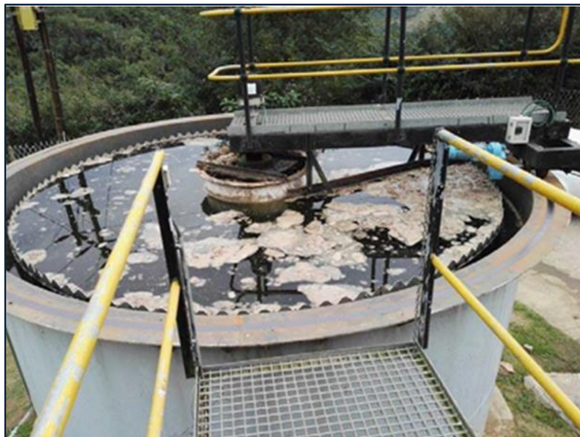
Figure 19.35 Camperdown Clarifier No. 2.
