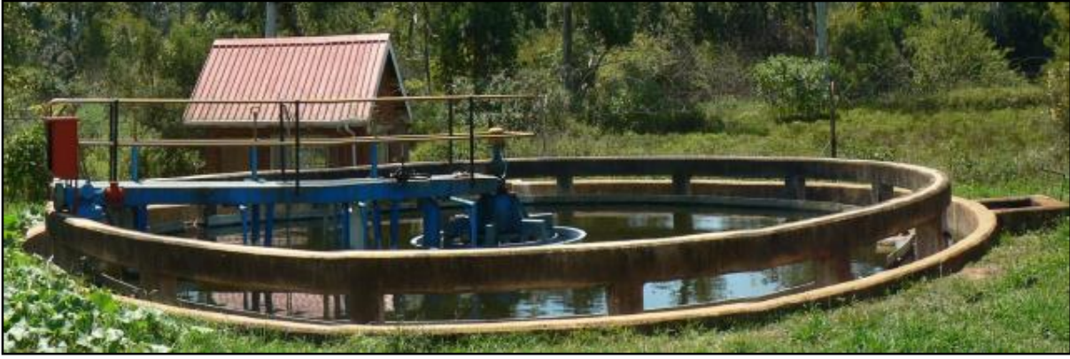
Figure 19.37 Richmond WWW clarifier.
