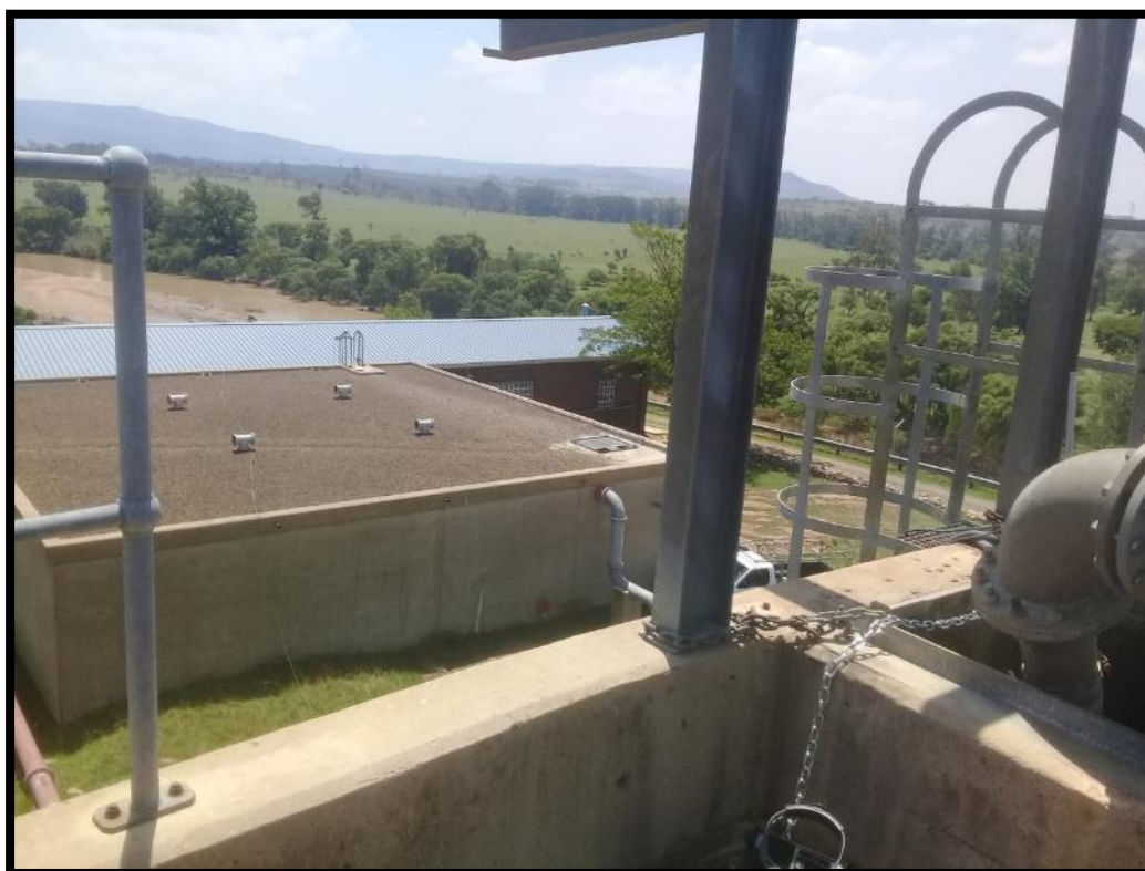
Figure 14.28 Photo of Vants Drift WTP (March 2020)
