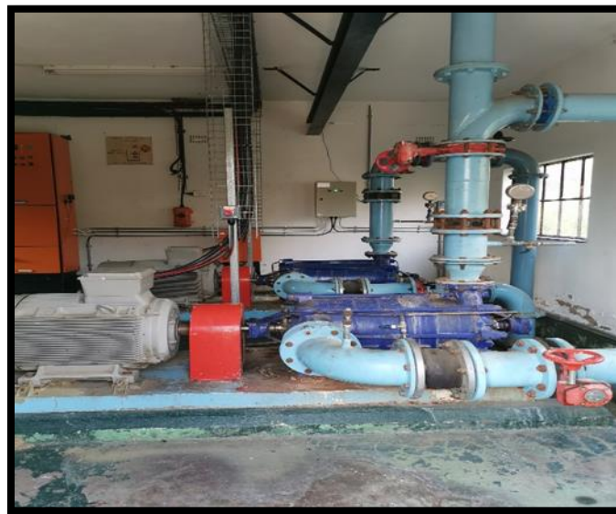
Figure 14.41 Utrecht Clear Water Pump Station
