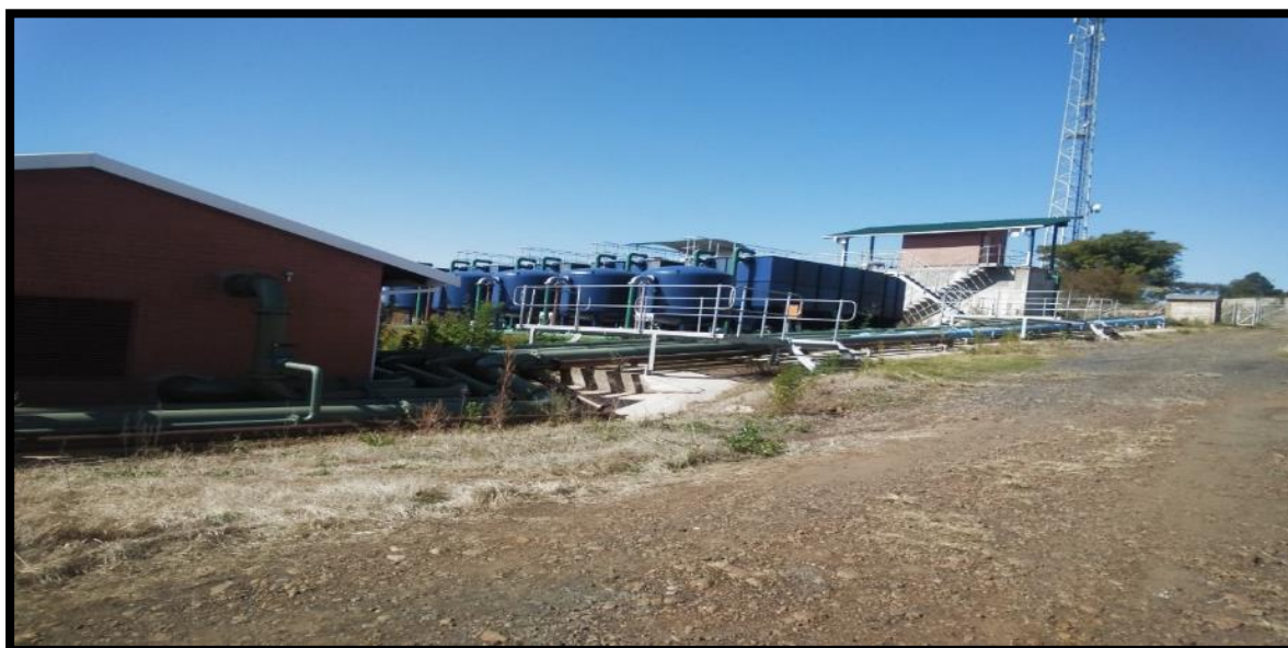
Figure 14.34 Photo of Durnacol Water Treatment Plant (May 2020).
