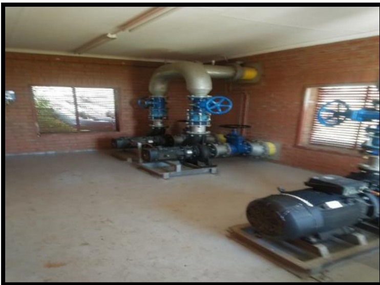
Figure 14.37 Durnacol Clear Water Pump Station (May 2020)
