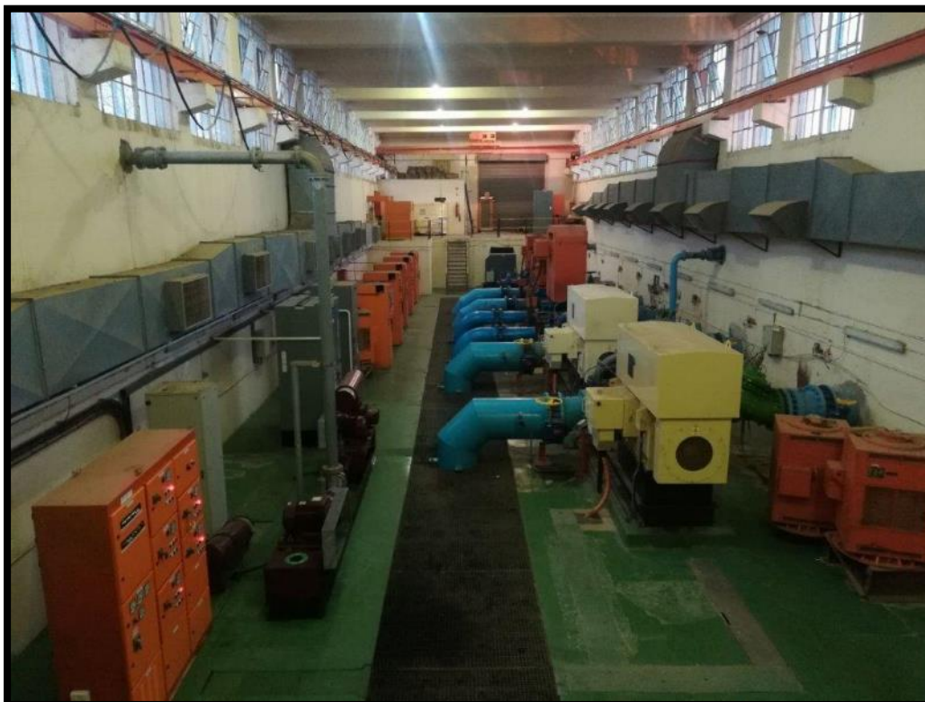
Figure 14.23 Photo of High Lift Pump Station at Ngagane WTP (May 2020)
