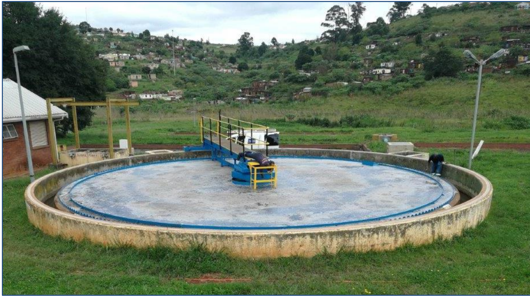
Figure 19.9 Clarifier No. 1 Ixopo WWW.
