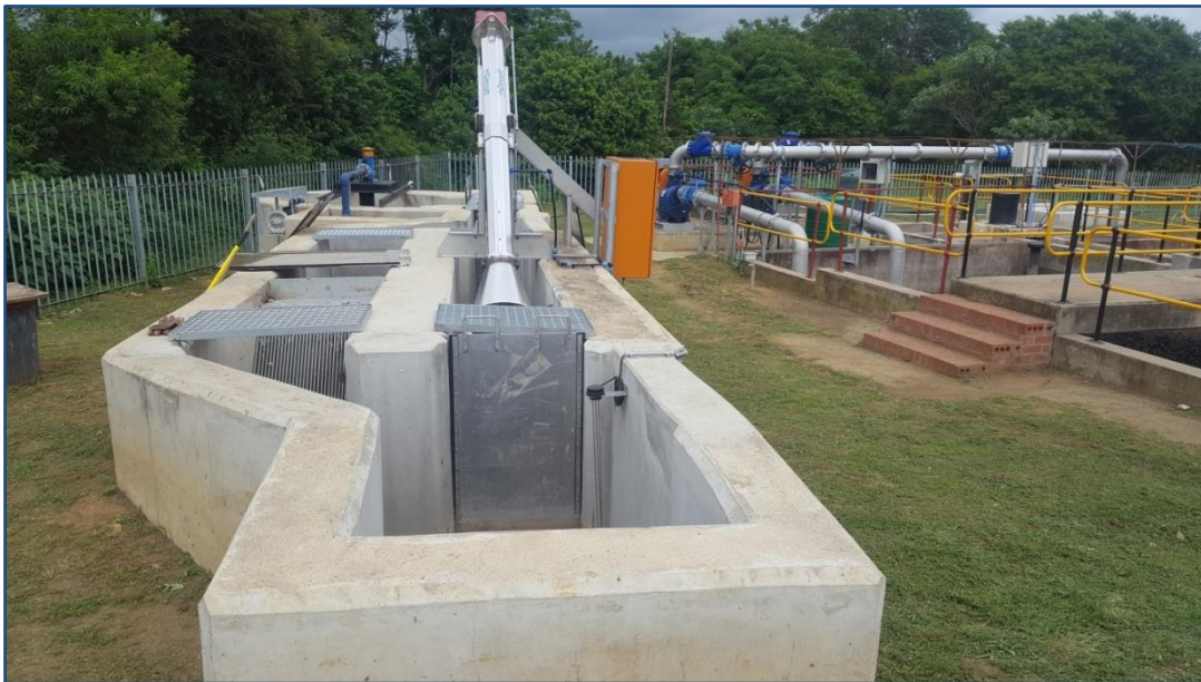
Figure 19.21 Lynnfield Park WWW head of works showing manual and mechanical screening channels.
