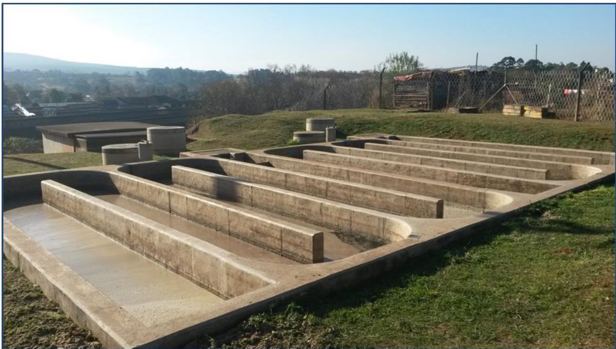
Figure 19.14 Howick WWW Chlorine Contact Tank.
