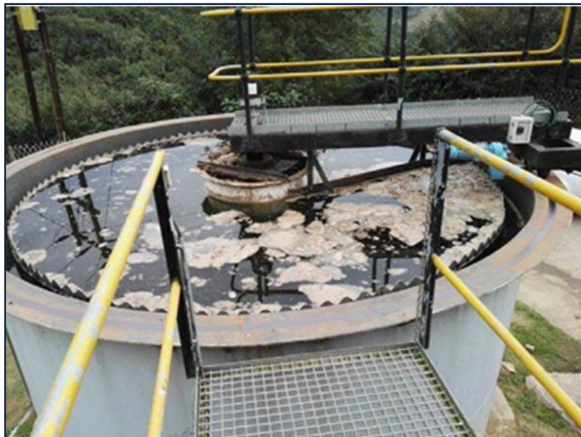
Figure 19.36 Camperdown Clarifier No. 2.
