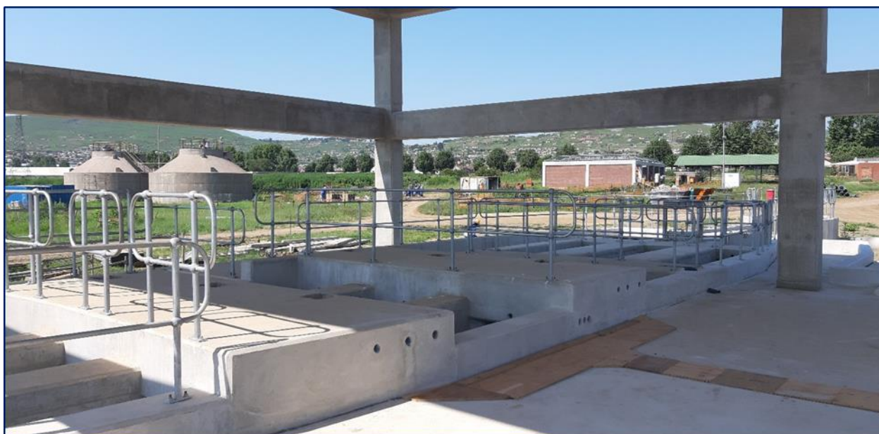
Figure 19.44: Mpophomeni Wastewater Works New Head of Works
