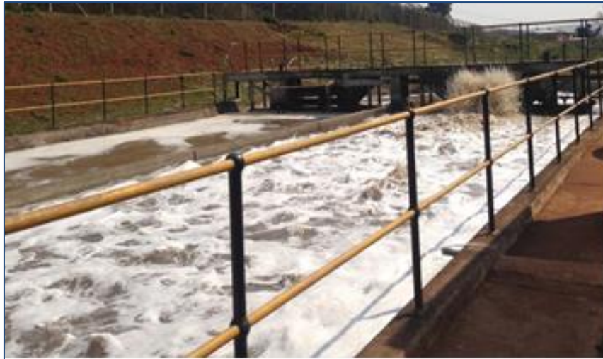
Figure 19.28 Appelsbosch WWT Oxidation Ditch (Aeration Tank).
