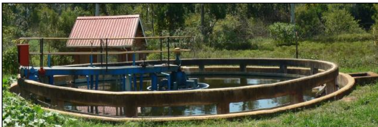
Figure 19.38 Richmond WWW clarifier.
