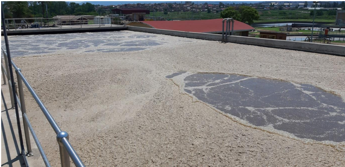
Figure 19.7 Darvill Aeration Basin.
